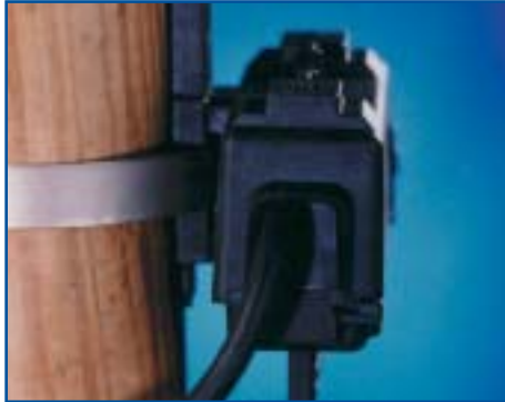
Single pole unit strapped to pole
