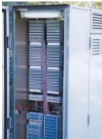
Digital loop carrier applications utilising HIGHBAND 10 for customer distribution with over voltage and over current protection and HIGHBAND 20 for density. Also xDSL applications.
