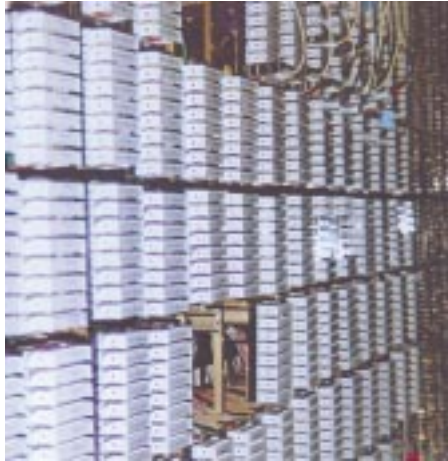
Digital Distribution Frame application for high density 64 twisted pair circuits instead of co-axial cable. HIGHBAND Compact 8 modules are utilised.
