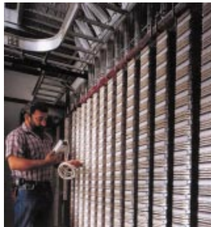
Building distribution utilising HIGHBAND 10 structured cabling ie. fibre to the building applications.
