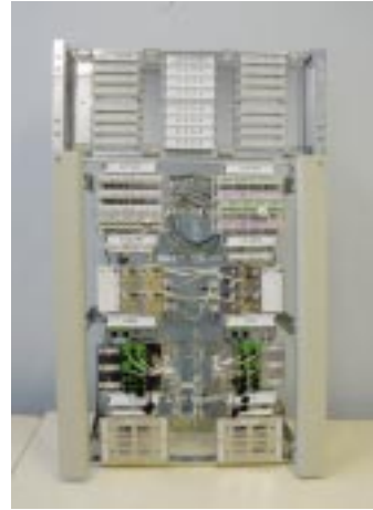
POI Point of Interconnect. Application is the termination of various media including twisted pair on HIGHBAND 10. Small station DDF's 19" rackmount with HIGHBAND Compact 8. Fibre and coaxial termination on the one KRONE mounting frame.
